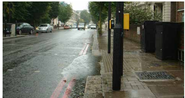
Water 'ponding' at a controlled crossing due to poor design and detailing of drainage.
