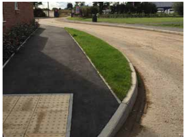
This small grassed verge serves little purpose and creates a maintenance burden.
